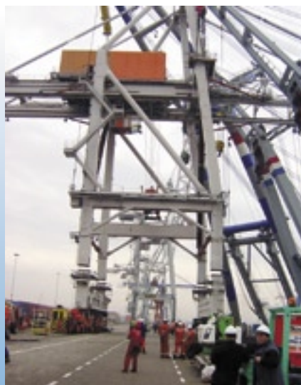
Lifting the crane. The 'splitting-point' of the legs is the lower part of the extension pieces.
