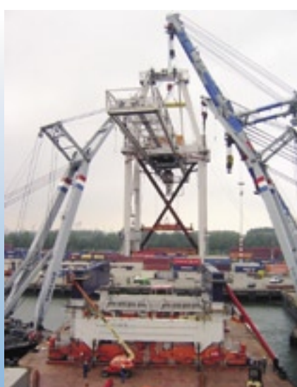
The pontoon is being manoeuvred underneath the crane. The bogies on rails on deck of the pontoon. The new blue portal beams that span 20m.
